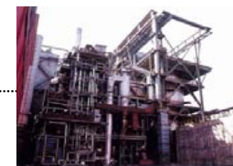
Coke dry quenching equipment (CDQ)
